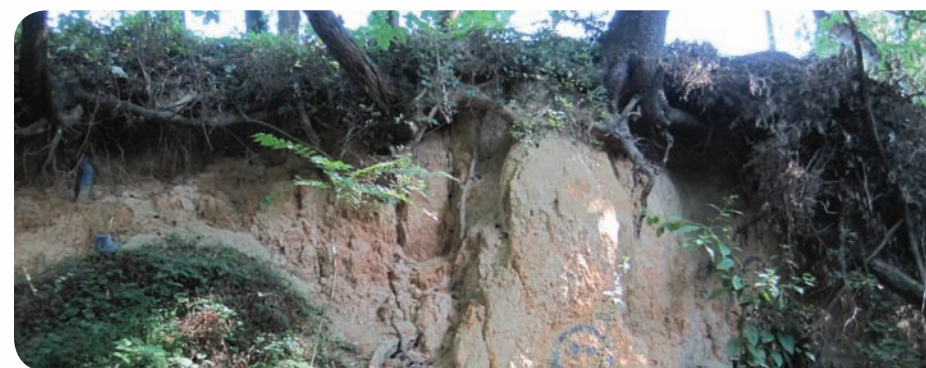
Steep slopes, like the side slope shown above, exist in several areas along the rail trail corridor.
