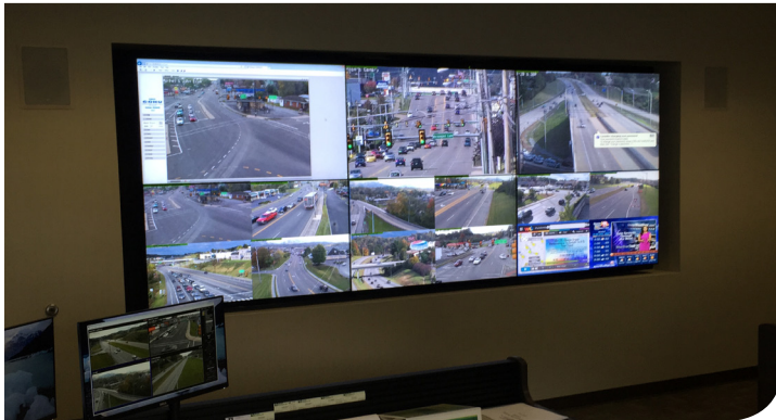
Traffic Operations Center
